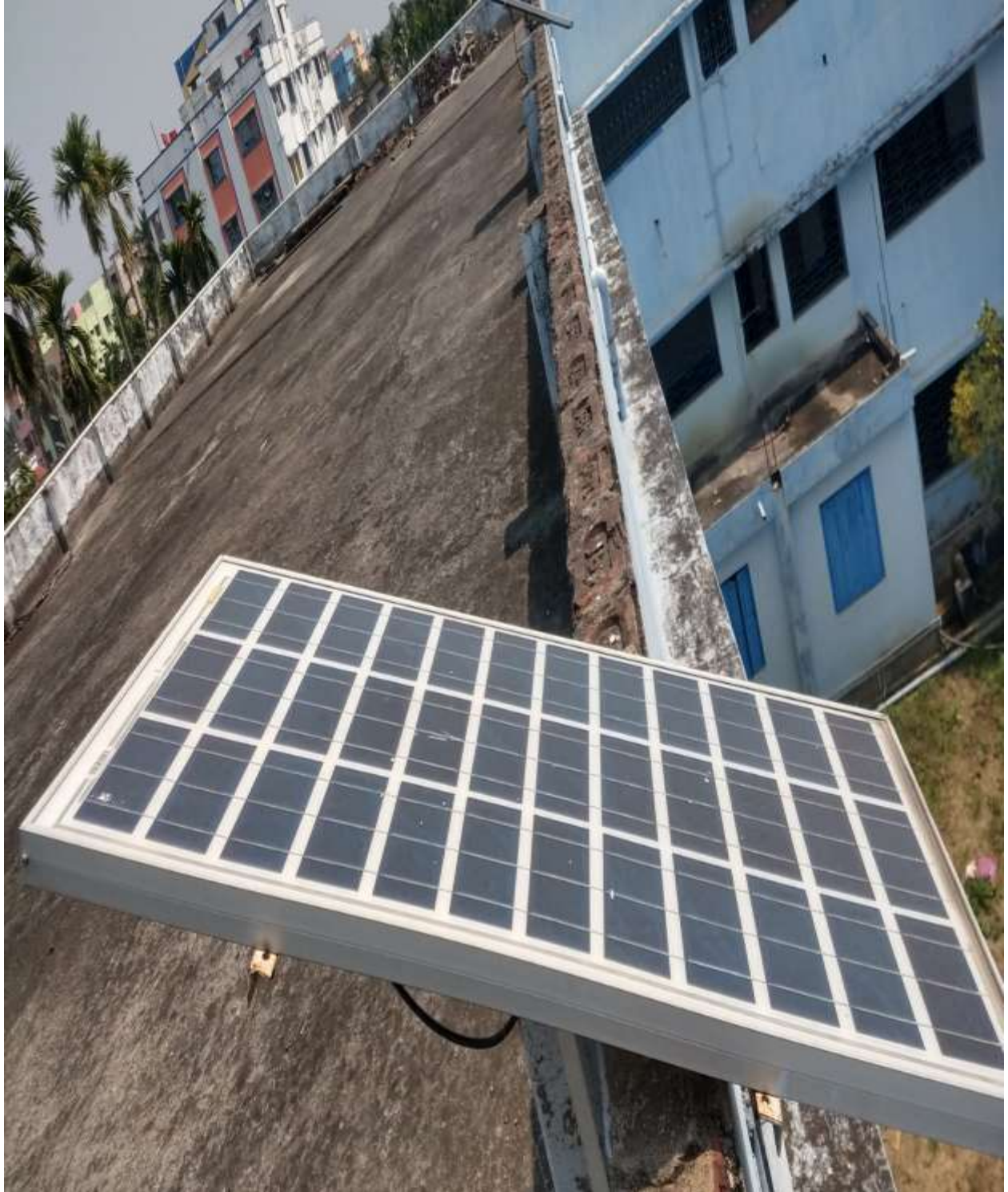
Solar Panels planted on the roof of the college
