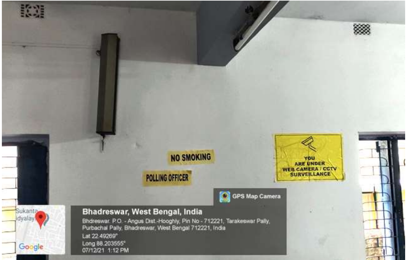
ROOM NO-1 Sound System, CCTV
